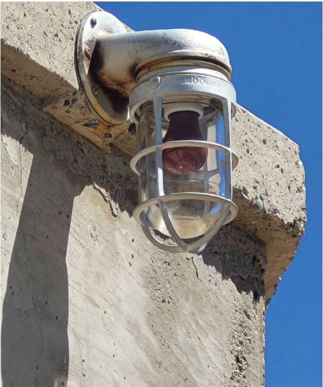
Fig 9. Photographs of the existing fixtures at the Cerro Tololo (AURA-NOIRLab) facilities.
